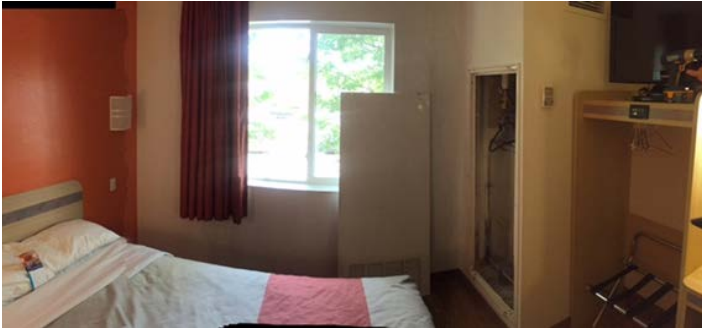
Interior of a Motel 6 room; on the right, the access panel has been removed to show the enclosure for the VPAC unit.
