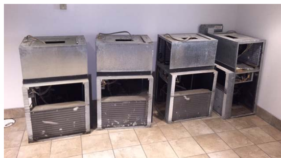
Seen here, the previous VPAC units await their removal from the Motel 6 site in preparation for the new VPAC unit installations.
